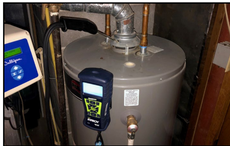
Image 4. Technician measuring undiluted carbon monoxide with a combustion analyzer after performing the steps outlined above.
